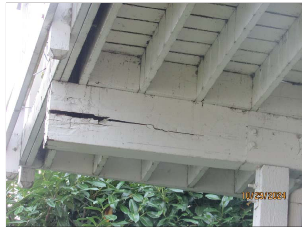
DAMAGED BEAM UNDER DECK
